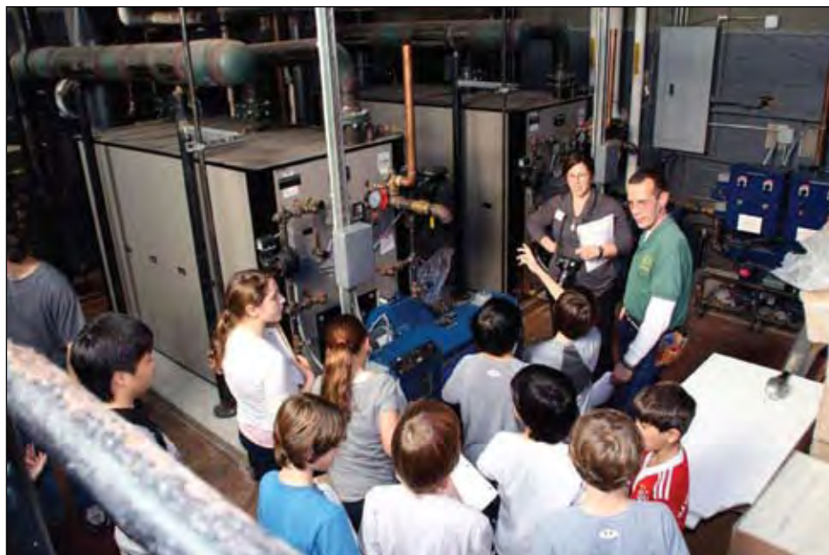
Pleasantville Middle School sixth-graders visited their school's boiler room, one of several places where they learned about the building's ecological footprint and issues that affect the environment.
